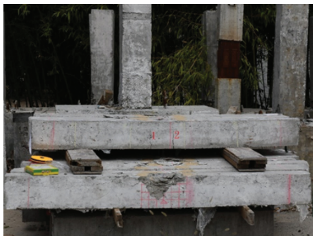
Figure 1: Concrete beam specimens with cracks on surface
