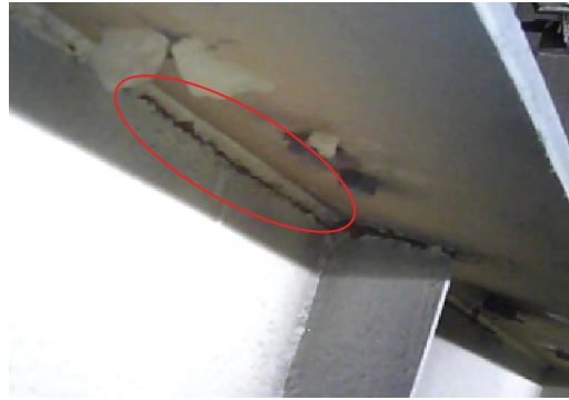
Figure 1: A failed steel CRG due to a surface crack at the weld joint between the upper flange and web plate
