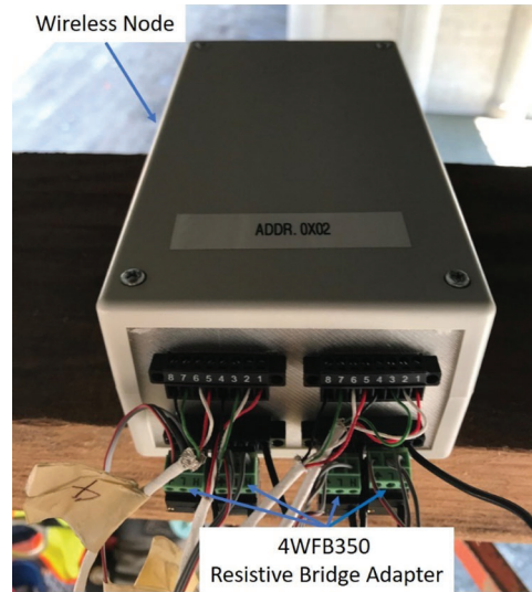
Figure 14: Resistive bridge adapters connected between wireless node and sensors
