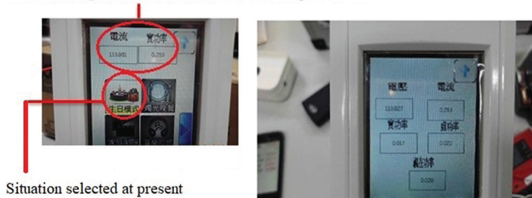
Figure 12: Touch human-machine interface display of an electric meter
