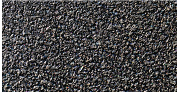
Figure 9: Rough asphalt pavement
