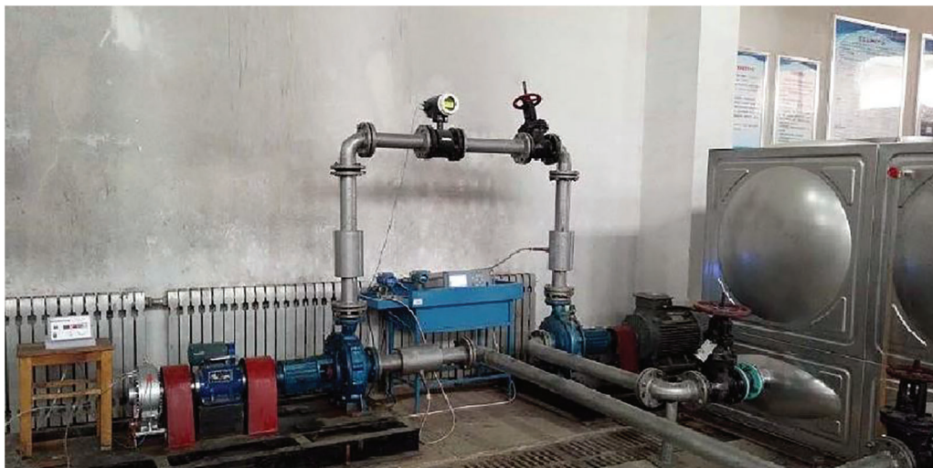
Figure 7: Hydraulic turbine test bench
