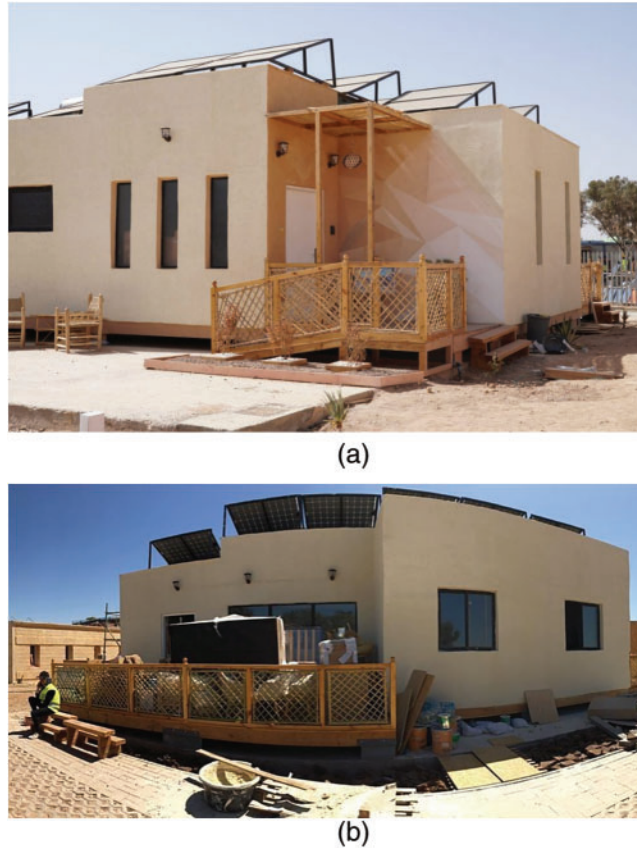
Figure 7: (a) The installation of the photovoltaic system in the roof of A'freehome in the south façade; (b) The installation of the photovoltaic system in the roof of A'freehome in the north façade
