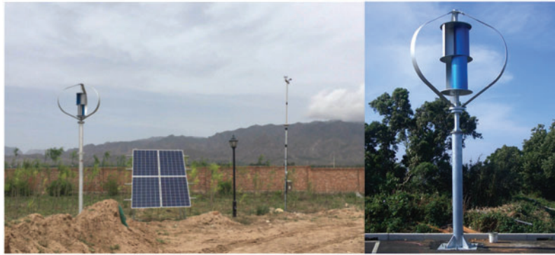
Figure 1: Example of decentralized wind power generation (test site live shooting)
