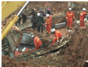
(a) #GuangmingLandslide#It's happening quickly!! Just 5 meters away from a miracle of life! According to on-site reporters, the image now shows the fourth floor, and signs of life are on the first or second floor!! Go, Zhongshan Fire Rescue Team!!! (Reporter: Jiang Tianli)
