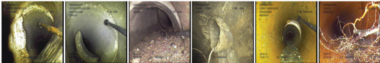
Figure 1: Photos of underground pipe defects
