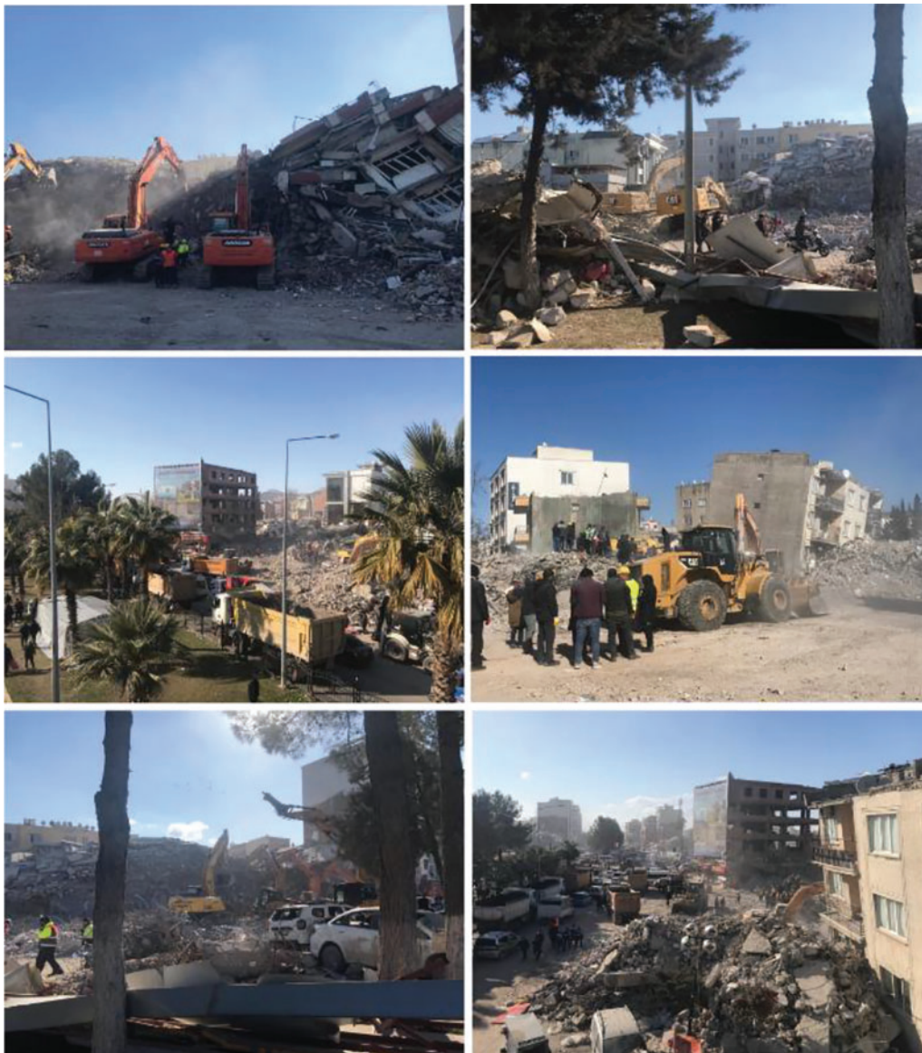
Figure 5: Debris removal after the earthquake in the Adiyaman City
